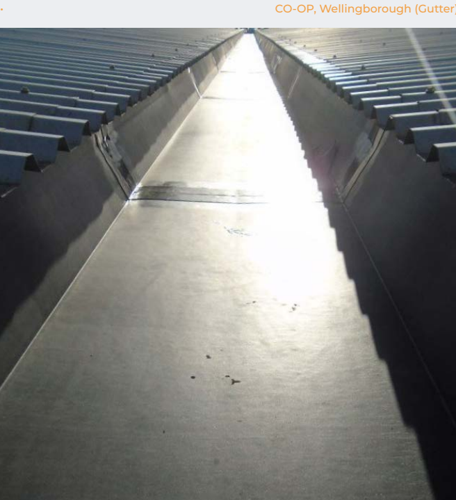
CO-OP, Wellingborough (Gutter)
